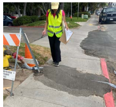
Figure 6. Pipe coming from the fire hydrant that has been paved over disrupting the sidewalk and curb
