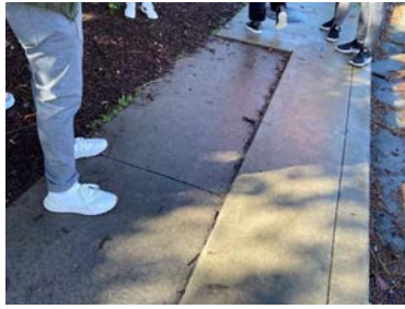
Figure 4. Lifted sidewalks along Naples St. between Broadway & Industrial Blvd.
