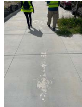
Figure 6. Bike path and walkway are not clearly marked.
