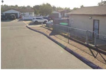
Figure 1. Dirt path that leads to Loma Verde Elementary from Loma Ln. needs pavement and maintenance.
