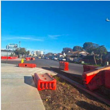
Figure 4. Construction barriers knocked down at the corner of Orange Ave. & 39th St.
