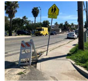
Figure 4. Curb ramp at the corner of S. 40th St. & Z St. needs maintenance
