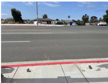
Figure 4. Missing "no pedestrian crossing" sign.
