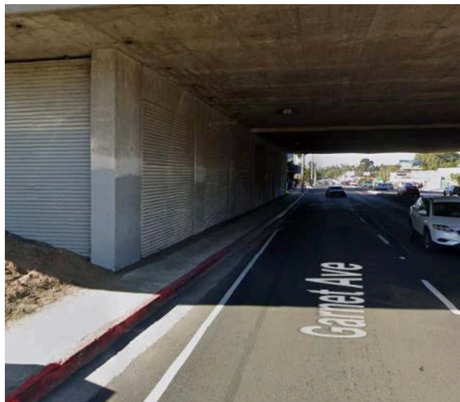
Figure 7: Photo of poorly lit and narrow sidewalk I-5 underpass on Garnet Ave.
