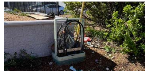
Figure 2. Exposed electric boxes on Oxford St. between Broadway & Industrial Blvd.
