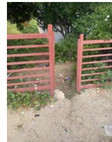
Figure 1. Wobbly Fence (between Naranja St. and Groveland Dr.)
