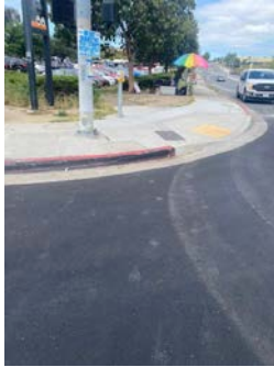
Figure 3. Needs additional curb cut (SW and SE corners of Euclid Ave./Market St.)
