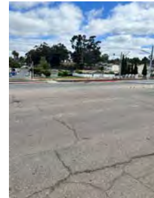
Figure 7. Labeled crosswalks are needed along Imperial Ave. that connects the trolley stop to the main sidewalk
