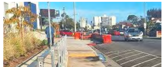
Figure 2. Handicap ramp needs repair in front of Central Elementary on Orange Ave. between 37th St. & 39th St.
