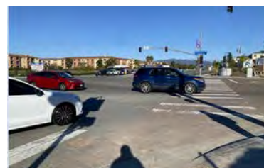
Figure 3. Crosswalks on intersection between Caliente Ave. & Otay Mesa Rd. need to be repainted.
