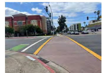
Figure 2. Curb not cut on Market St. and 47th St.
