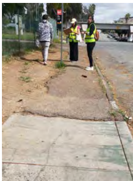
Figure 4. Sidewalk ends at entrance to 47th St. Trolley Station
