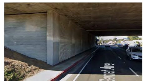
Figure 3. I-5 underpass on Garnet Ave. contains narrow sidewalks, debris, and poor lighting
