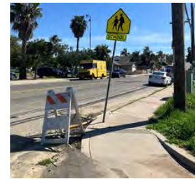
Figure 4. Curb ramp at the corner of S. 40th St. & Z St. needs maintenance
