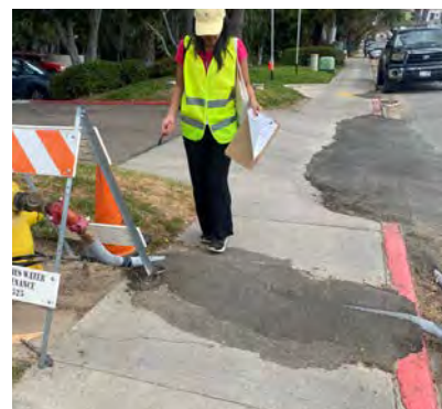
Figure 6. Pipe coming from the fire hydrant that has been paved over disrupting the sidewalk and curb
