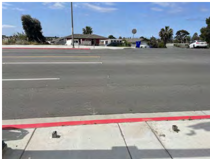
Figure 4. Missing “no pedestrian crossing” sign.
