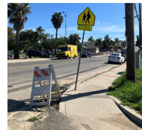
Curb ramp at the corner of S 40th St & Z St needs maintenance
